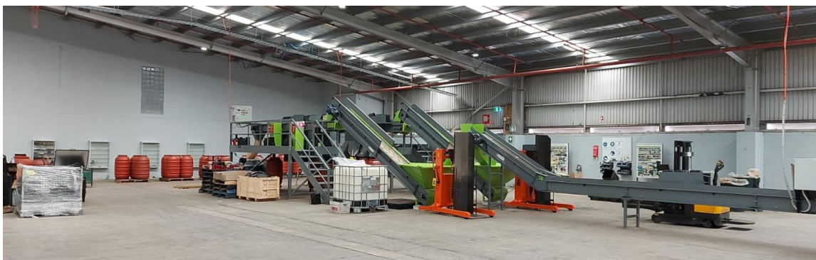
Sorting equipment in situ at the Laverton site.
